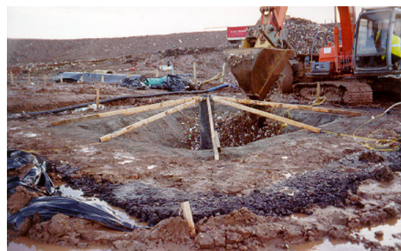
Figure 5 Completed experimental liner system prior to filling and fitting of the rain cover
