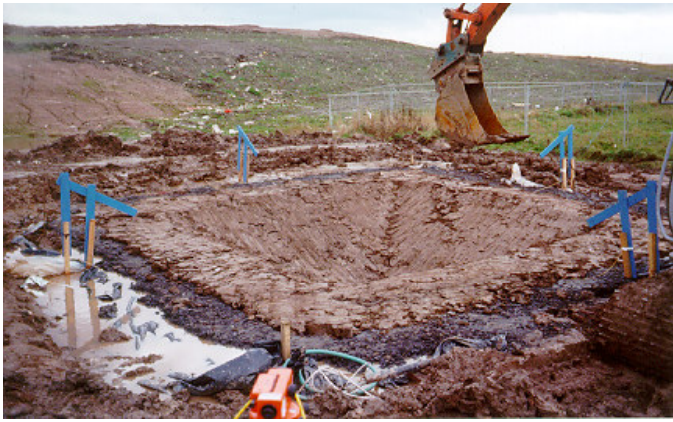
Figure 10 Compaction of the clay on the surface of the lower concrete layer.
